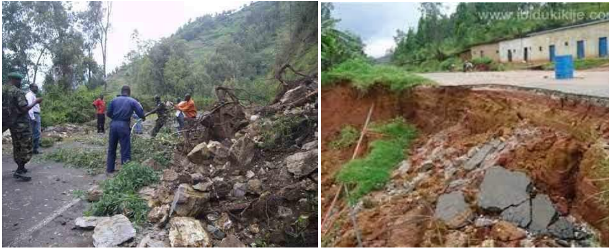
Figure 7. Landslides caused by manmade works (Roads), Ngororero and Rubavu.
