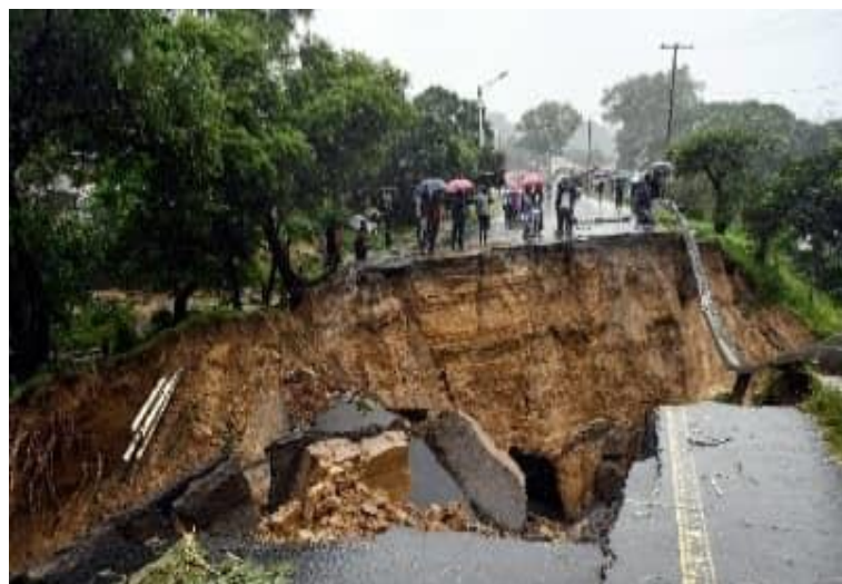
Figure 4. Road destruction in Rubavu.
