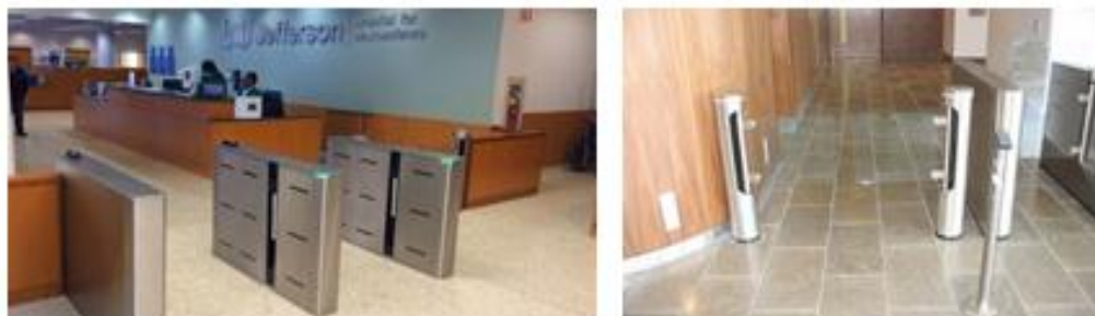
Figure-3. Access Control System
