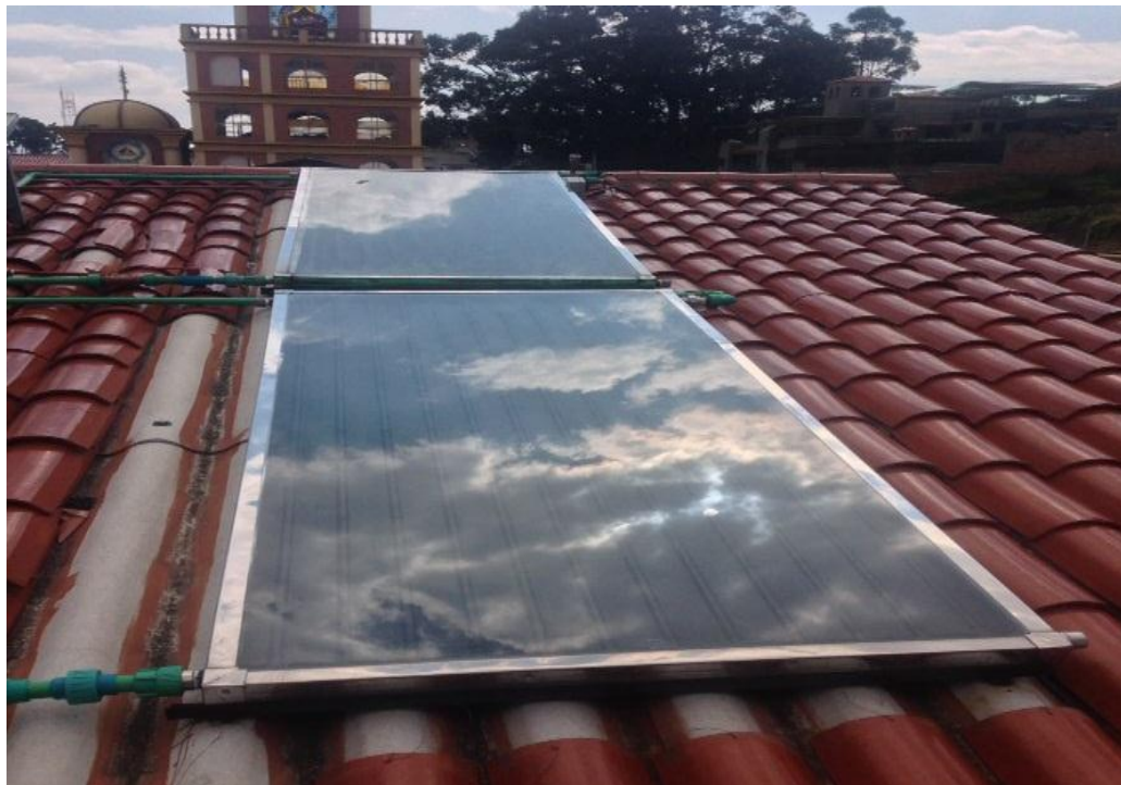
Figure-1b. Thermal solar panel.
