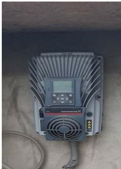
Figure-4. Variable frequency drive.
