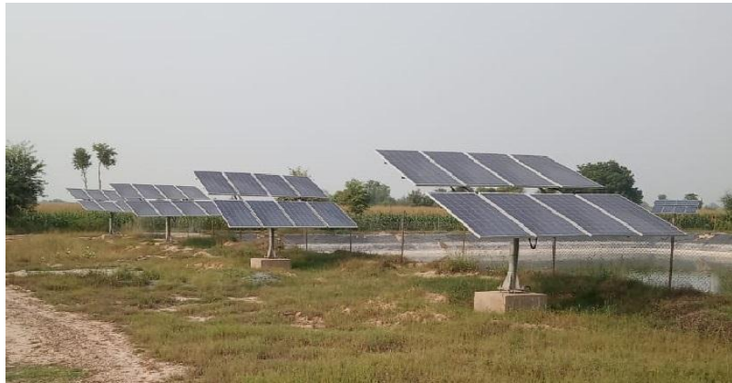
Figure-3. Installed PV System on Site.
