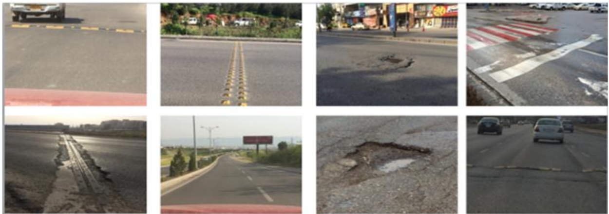
Fig-6. Diverse street samples (showing normal speed bumps, manholes, potholes, etc. ) Photos were taken by the others in the cities of Sulaimaniyah and Erbil (North of Iraq).
