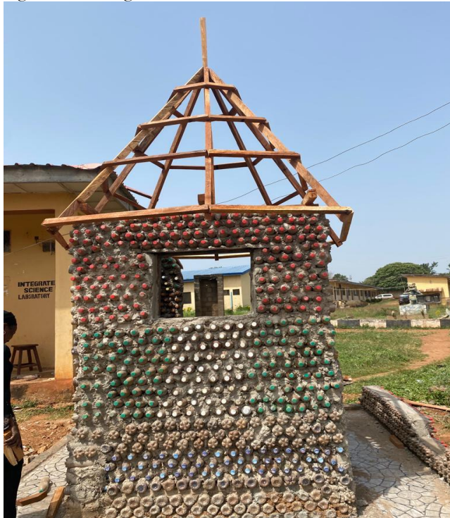
Stage Eight: underlying the grass roof with nylon to prevent water from entering during raining season
