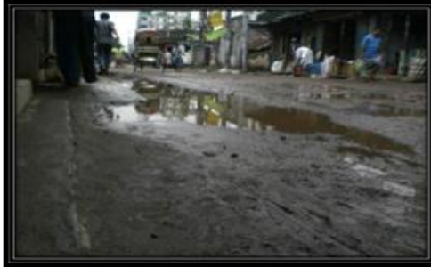
Figure-7. Water Logging
