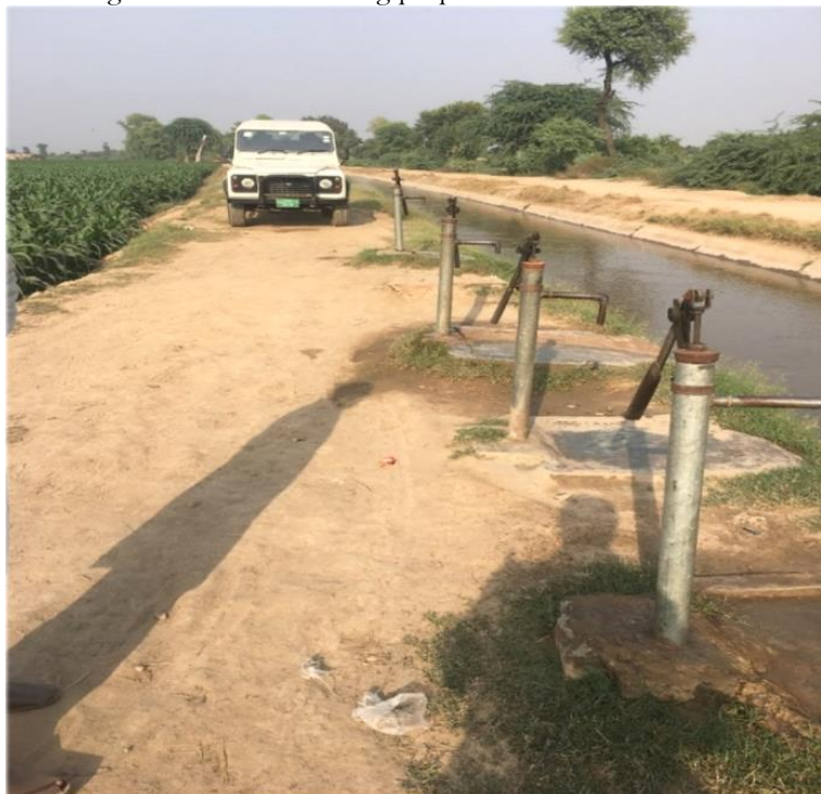
Figure 7. Hand Pumps installed on Nasrana canal for drinking water.
