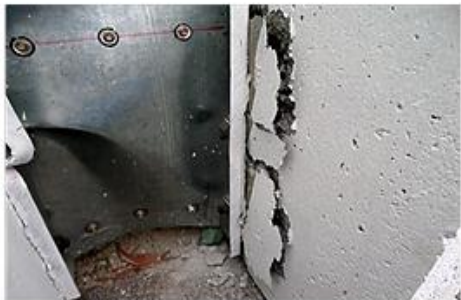
(c) Crushing of concrete
