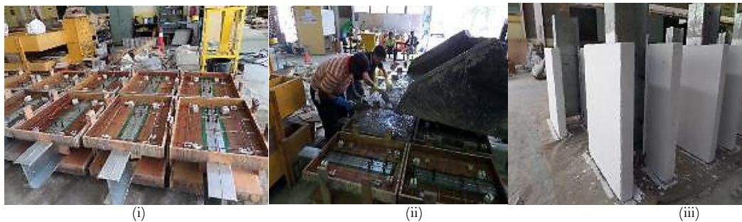
Figure-1. Preparation of test specimens [(i) Formwork, (ii) Casting, (iii) Finished samples]
