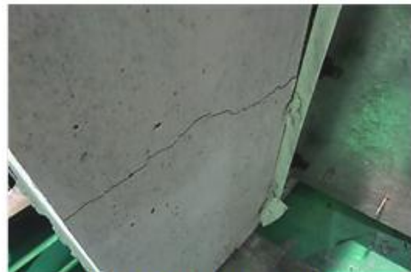
(b) Cracks underneath slab
