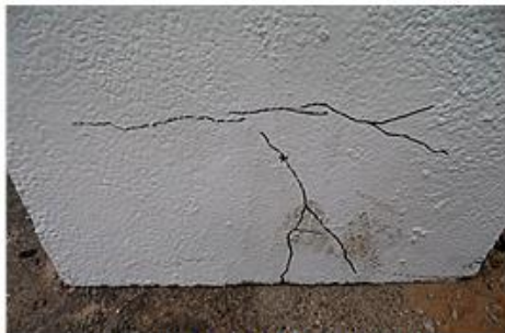
(a) Surface cracks on slab
