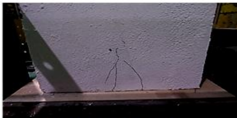
(a) Cracks on slab surface
