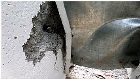
(c) Crushing of concrete
