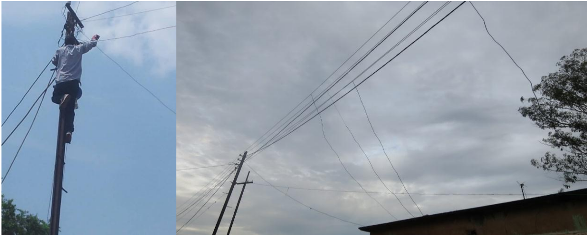
Figure-1. Case of the theft of electricity by connecting to the air network in Lubumbashi.
