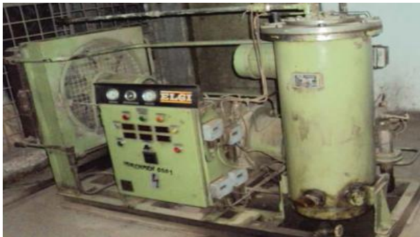
Air Compressor (Imported from India)
