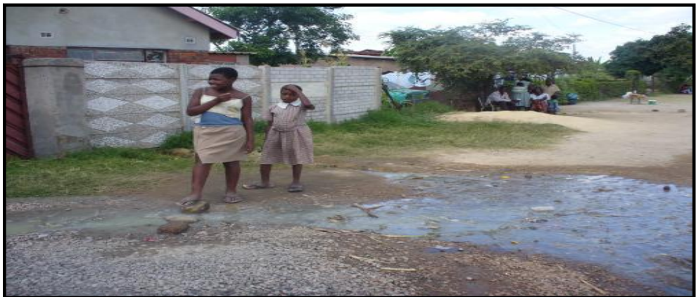
Figure-4. Sewerage system failures in Harare
