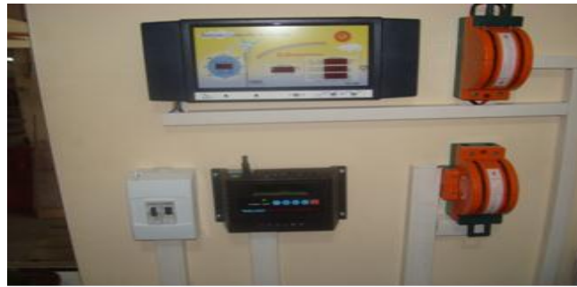
Figure-5. The general view of the controller
