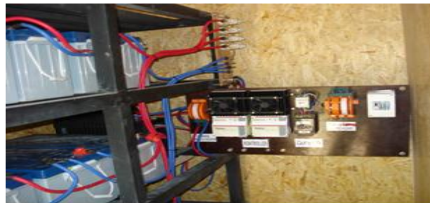
Figure-6. The general view of the accumulator system
