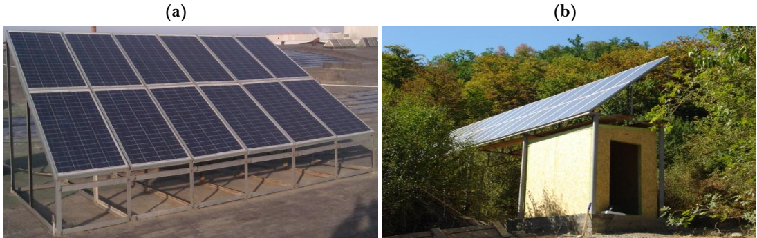
Figure-4. The general view of the solar panels, ((a) – in Baku city, (b) – in Gusar region).
