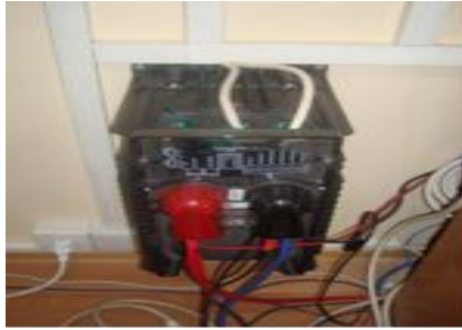
Figure-7. The general view of constant/ alternating current transformer.
