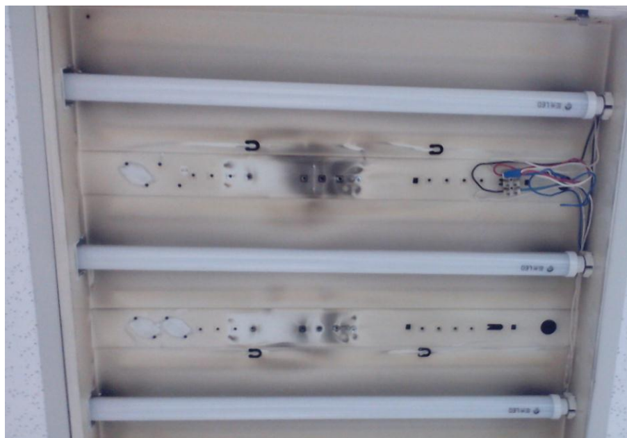
Figure-2. Florescent Fixture Modified to Accomodate LED's
