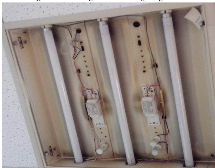
Figure-1. Existing Florescent Lighting Fixture
