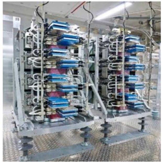
Fig-1b. A photo of installed MOS-FET
