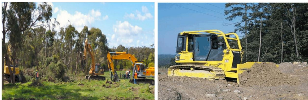
Plate-5. Bulldozer bringing down forest trees and removal of topsoil for quarry site
