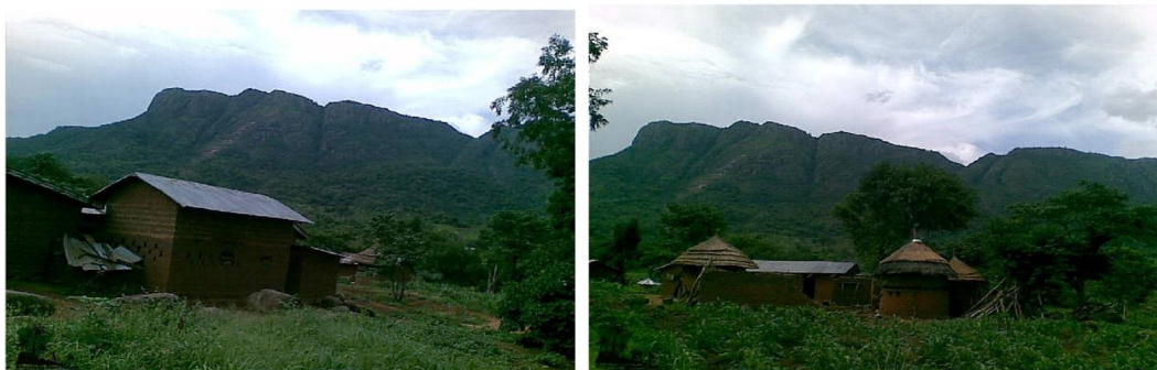
Plate-4. dilapidated buildings residing by indigents of the mine and quarried communities
