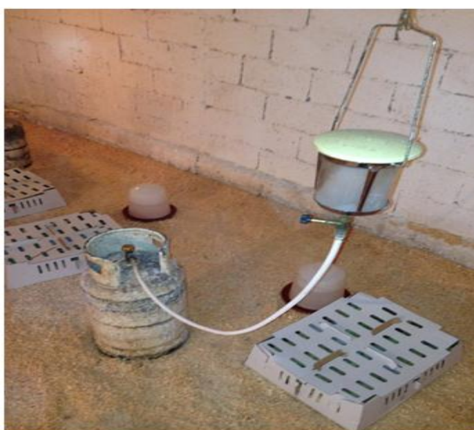
Figure-3. Gasoil heater with thermostat.
